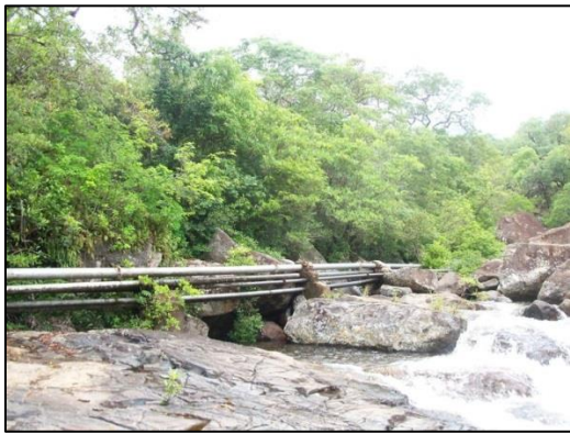
Figure 3.5: Water pipes on Mt. Mulanje in rains
